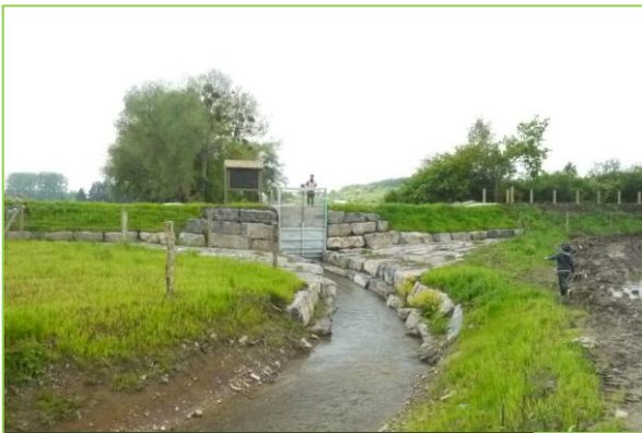
New infrastructure to control discharges including a gate and a low-water bed in order to facilitate fish migration
